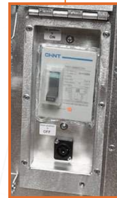
Inside view of breaker switch box
