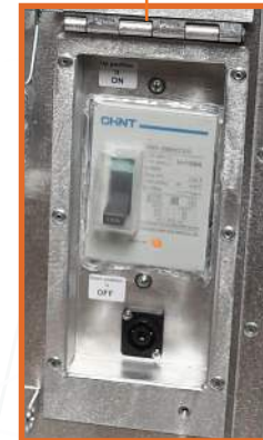
Inside view of breaker switch box
