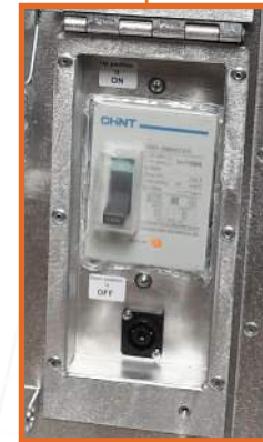
Inside view of breaker switch box
